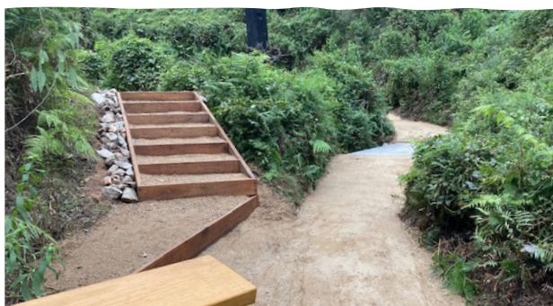
Images: Installation of steps, and finished product, at Fairy Dell Flora Reserve
